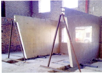
A wall panel in place and the light reflecting off the panel from the window opening, as well as an unpolished panel alongside the polished panel.
