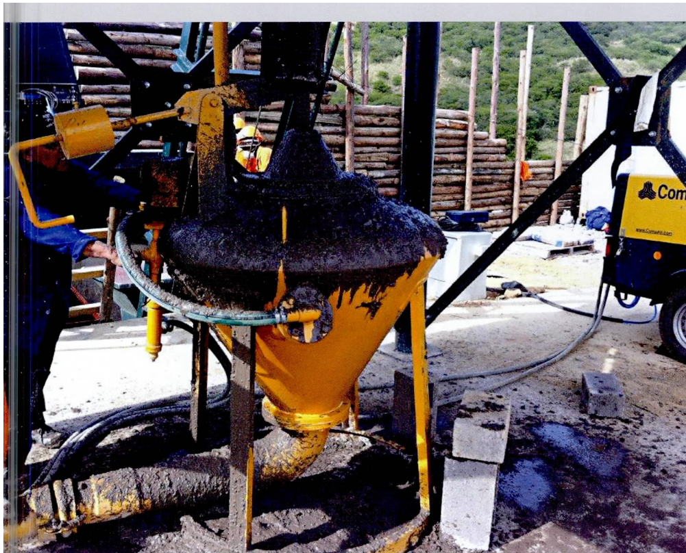
Sem 250 concrete placer pump in operation on a dam wall project in Umtata
