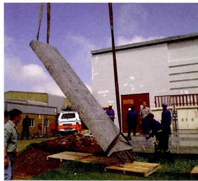
Use of an existing steel structure on the premises to create the PMSA showroom using pre-cast and pre-polished tilt-up concrete inner walls
