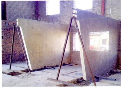
A wall panel in place and the light reflecting off the panel from the window opening, as well as an unpolished panel alongside the polished panel.
