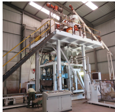
(Above): PA MSA RE1400 high-performance brick-making plant (Van Dyk Stene, Western Cape).
